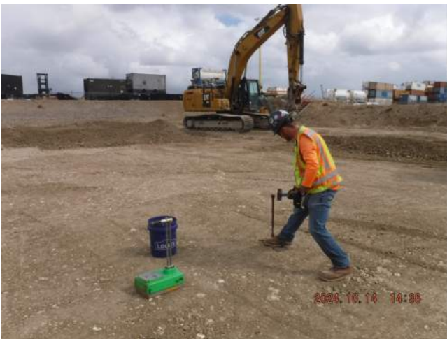
Pier 40F: MPE on site to take density tests of the compacted fill
