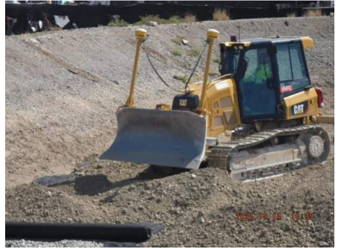
Pier 40F: KIWC civil crew (Sanu's) used the CAT D5 dozer to spread the fill placement in 12-inch loose lifts
