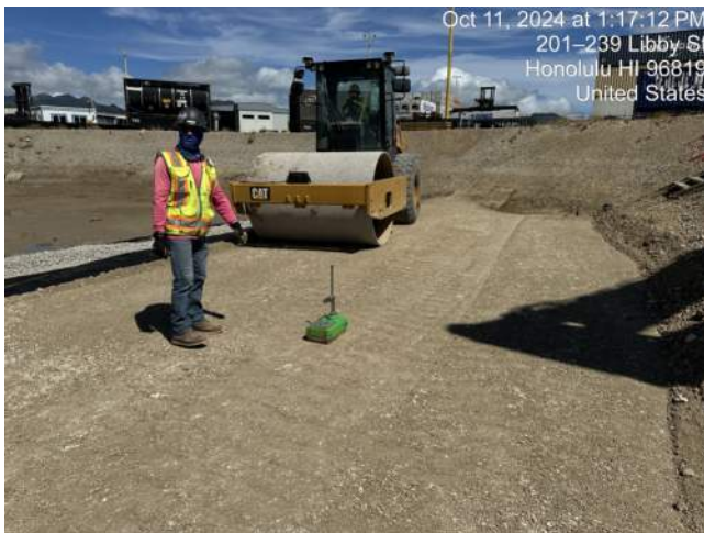
MPE testing compaction for the east section of "lane 1" in Pier 40F
