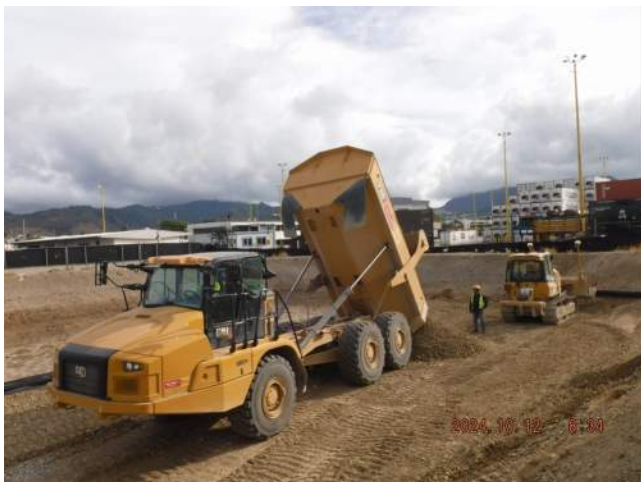
Pier 40F: The crew placed the minus (-) 3-inch crushed coralline material over the "burrito" wrapped grave
