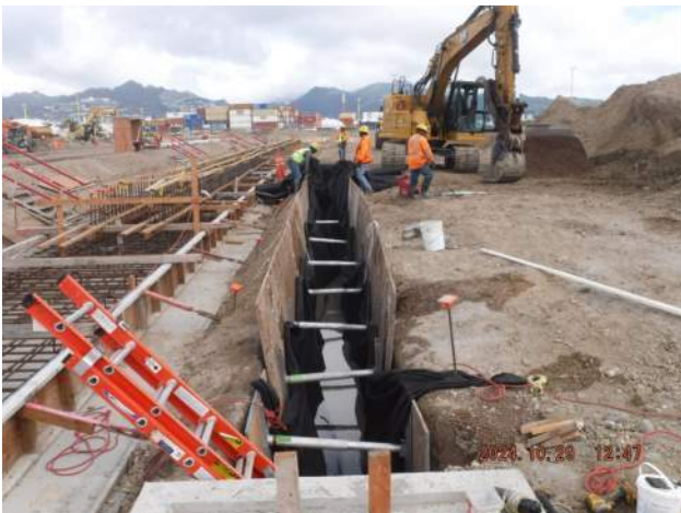
Pier 42: KIWC civil crew excavated the trench for SD 4 and installed the Mirafi fabric before placing the #3B fine gravel
