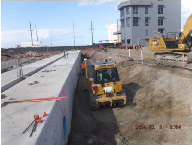
Pier 43: Backfilling, compacting and testing for P7 and P8 mauka of the LSCRB
