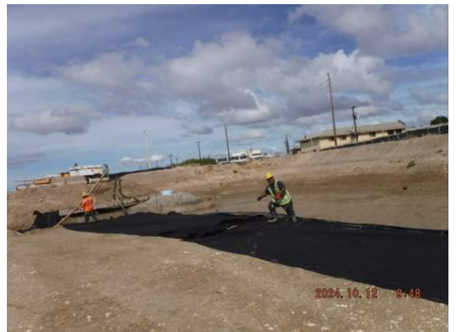
Pier 40F: The crew fused the 2 to 3 feet overlap of the Mirafi fabric before covering the bottom of the pond
