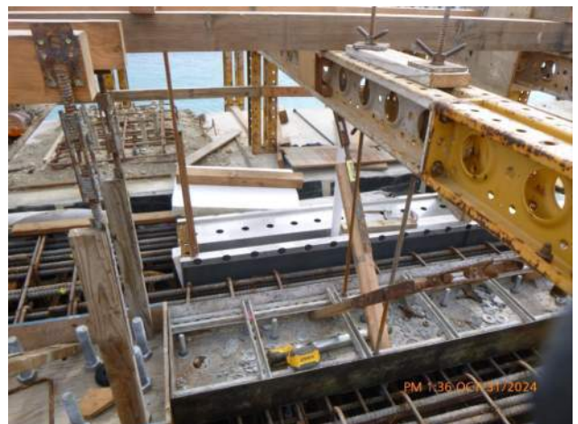
KIWC setting the crane rail pocket and cable trench hardware in WSCRB pour #A1.
