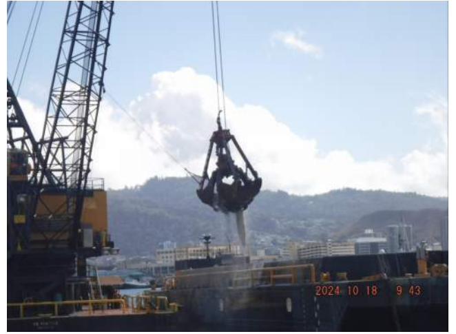
Pier 43: KIWC DB Seattle continued in water dredging between STA 8+60 and STA 6+00
