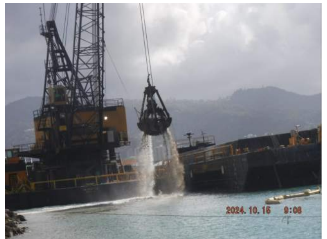
Pier 43: KIWC DB Seattle resumed in water dredging between STA 9+50 and STA 7+00
