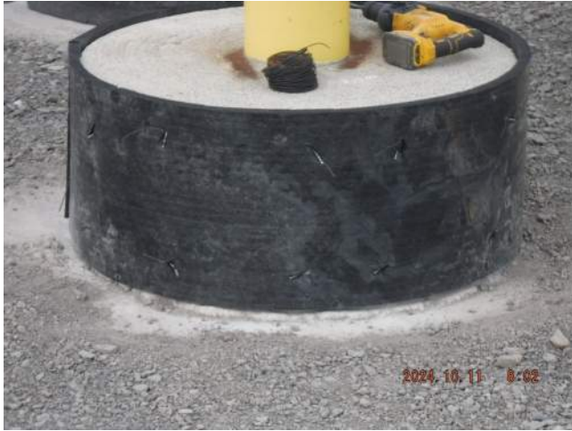
Pier 43: WL land 2 - KIWC foundation crew installed the 3/4-inch thick expansion board on the bases of the bollards
