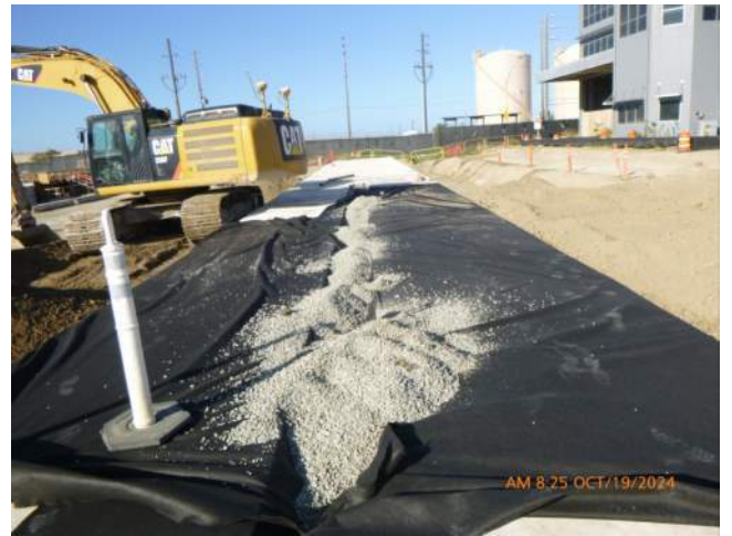
KIWC placing filter fabric and 3b in the LSCRb crane rail pocket.
