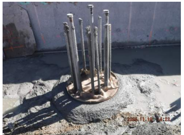
Pier 43: KIWC Foundation crew prepped the top of the concrete pour by placing the Sono tube covered with damp burlap material
