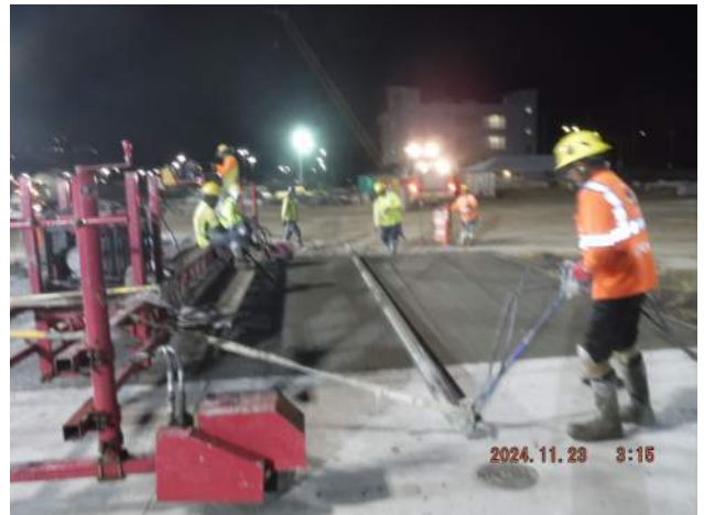
Pier 43: WMH Paving Block Out - KIWC crew used the Bunyan roller to level off the concrete pour
