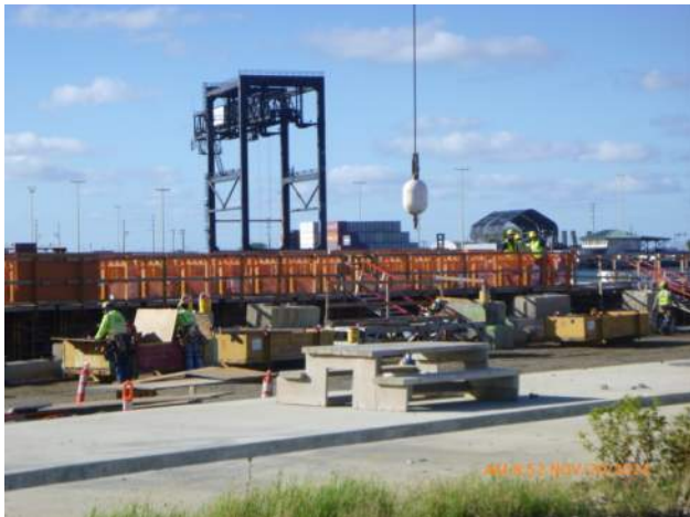
KIWC setting the blackout for the crane rail pocket in WSCRB pour #A2.
