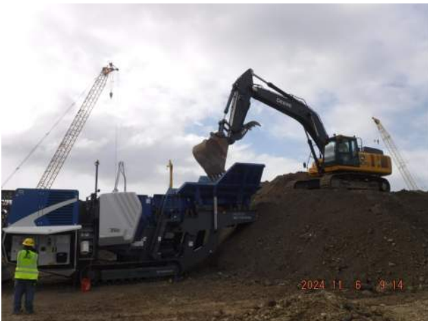
Pier 43: KIWC crew crushing the dredged material at the dredged material stockpile
