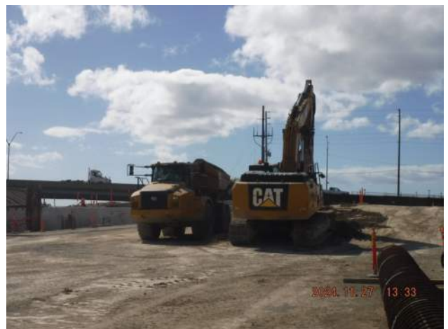
Pier 43: KIWC civil crew restored the ramp to its original width at the LSCRB over P7
