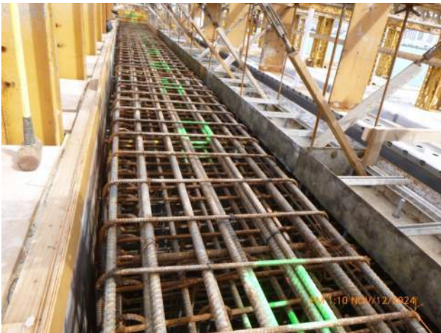
KIWC spreading rebar for concrete hose insertion into the WSCRB rebar cage.
