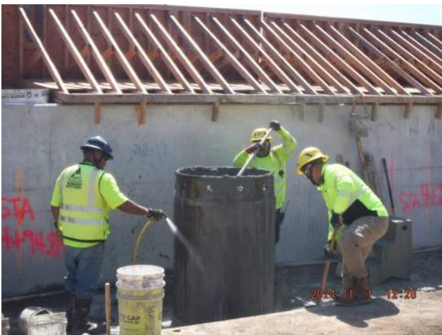
Pier 43: KIWC foundation crew continued to pull #3 casing and removed the concrete for placing the vibratory hammer
