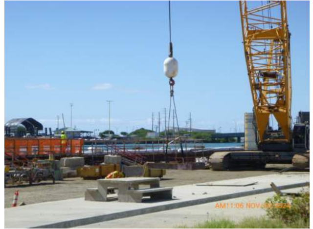
KIWC setting the blackout for the crane rail pocket in WSCRB pour #A2.
