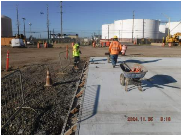
Pier 43: WL 1 and 2 block outs - KIWC paving crew stripped the forms of the PCCP blockouts
