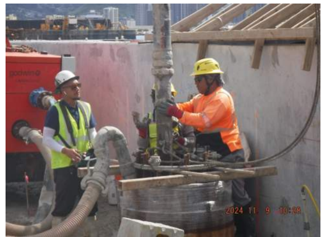
Pier 43: KIWC Foundation crew inserted the tremie pipe for the CIDH shaft 33-A1-36
