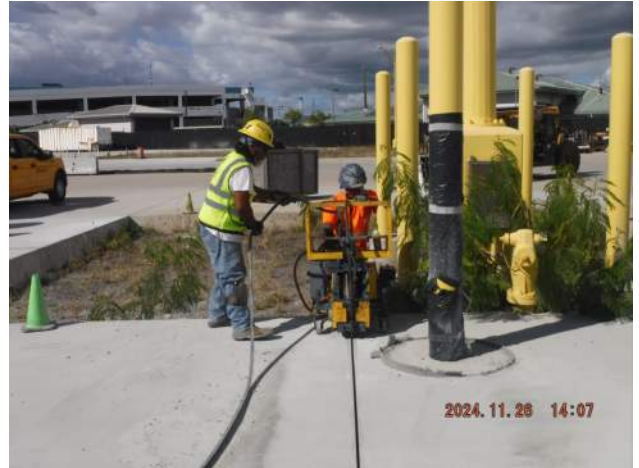
PCCP - KIWC paving crew continued to install the rubber sealant in the widened saw cut joints
