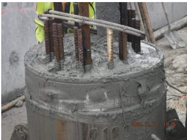
Pier 43: Concrete was allowed to overflow from top of the casing before pulling the first casing out
