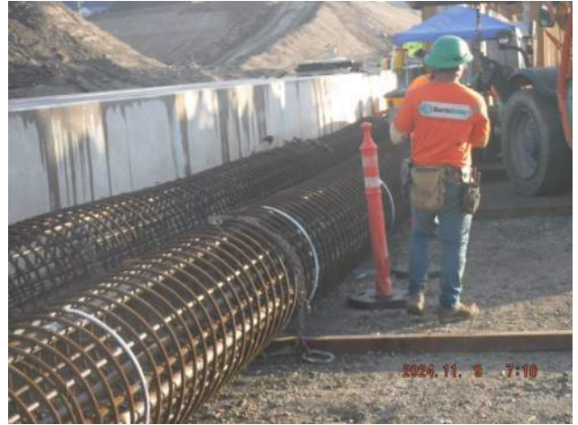
Pier 43: HRSPI crew on site to add rebar spirals for the 36-inch CIDH rebar cage
