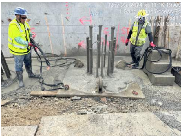
View of top of concrete in location 20-A2-36 after pulling remaining 5m of casing
