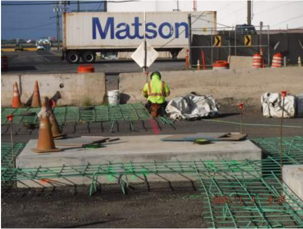
Pier 43: HRSPI continued to fabricate the rebar mat for the PCCP Block outs paving
