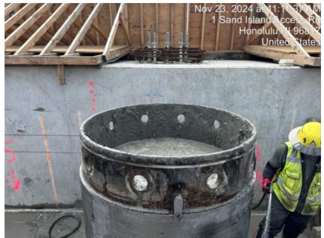
View of top of concrete in location 20-A2-36 prior to pulling remaining 5m of casing
