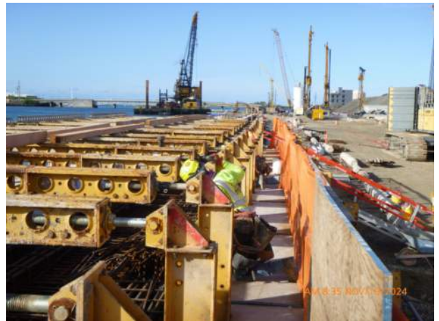
KIWC setting hardware for the crane cable trench in WSCRB pour #A2.
