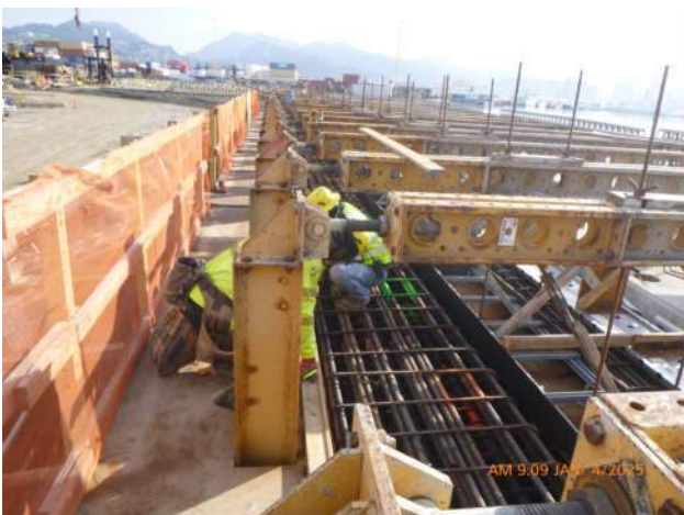
KIWC adjusting formwork around the bulkhead between WSCRB pours #A2 and A3.
