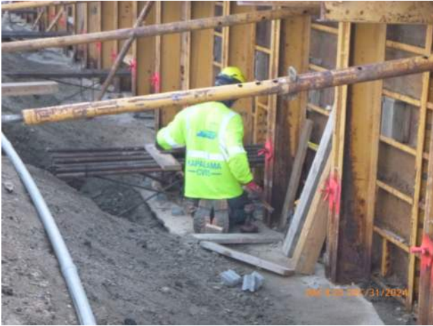
KIWC setting formwork around the embedded tie beam rebar in WSCRB pours #A1 and A2.
