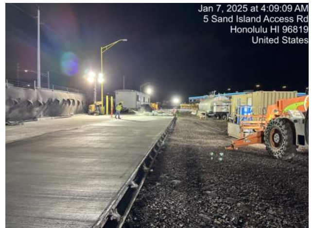
KIWC applying curing compound to the top of the freshly paved area
