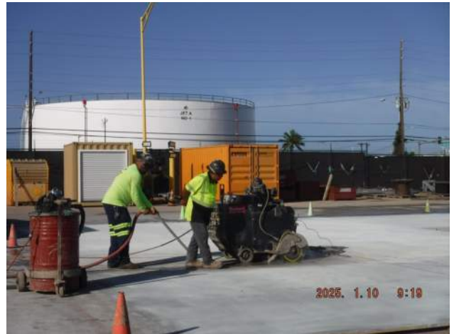
PCCP: MT3 - NCS crew on site to green saw cut the newly paved MT3
