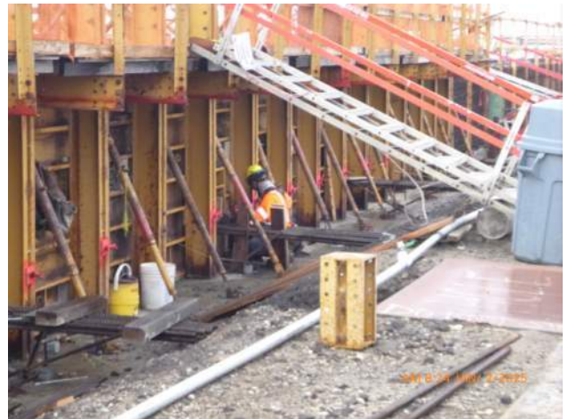
KIWC installing formwork around the embedded tie beam rebar in WSCRB pour #A3.
