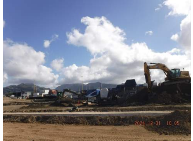
Pier 41: KIWC civil crew continued to crush the dredge material between STA 23+00 and STA 24+00
