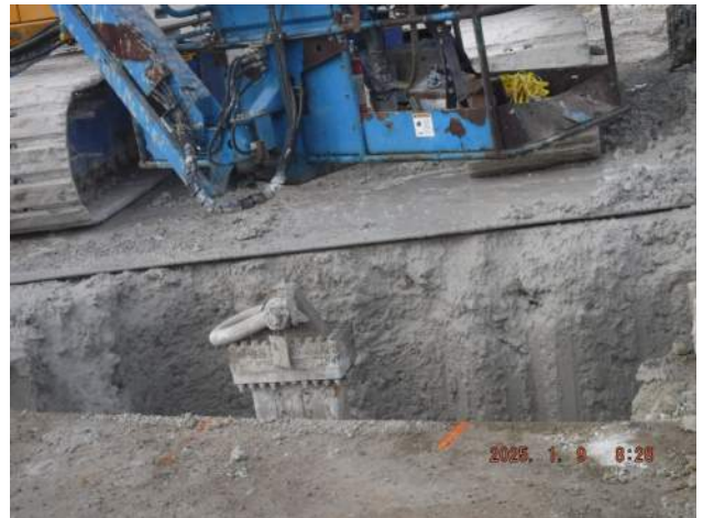
Pier 42: PF crew continued to drill around the cutter and the Kelly bar stuck in the ground in the junction structure
