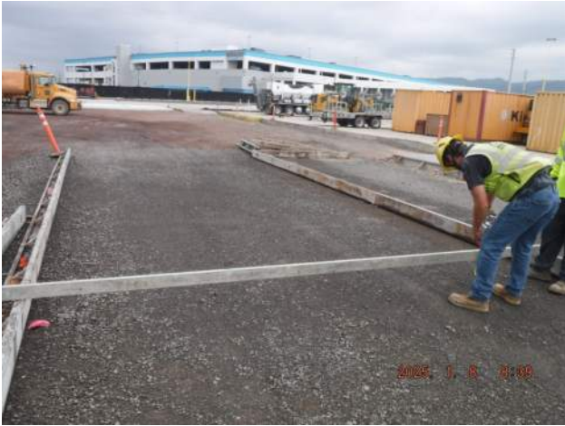
PCCP: KIWC and YKE crew grade checked MT 6 with grade issues. Recommended to fix the entire area before paving.
