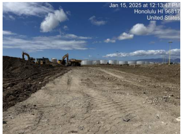
KIWC moving surcharge material to the crusher and the material storage bin north of the surcharge
