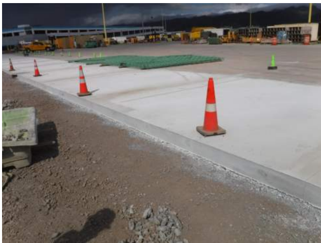
PCCP: KIWC paving crew sprayed the J9 concrete curing compound on the face of MT6
