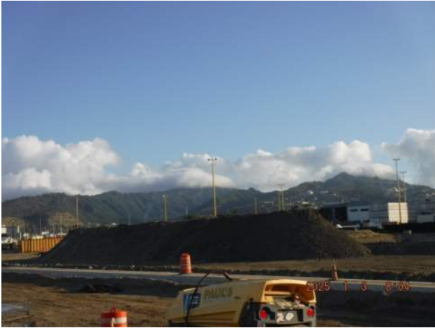
Pier 41: KIWC civil crew continued to stockpile the crushed material from STA 26+50 to STA 27+50
