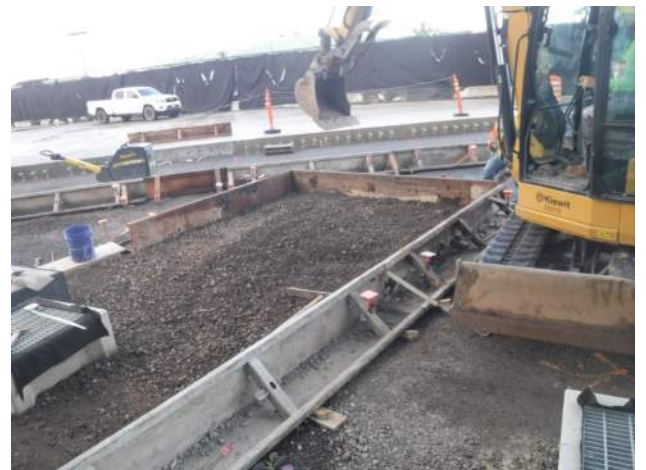
PCCP: PASHA maintenance - KIWC civil crew continued to grade and place basecourse aggregate for the block out
