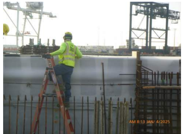
KIWC adjusting the 1/4" filler board on the wall of the CWCB next to the cable drum vault.
