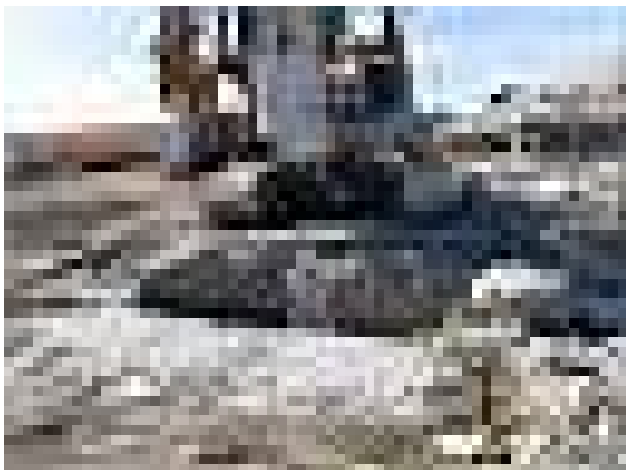
Pier 42: PF crew excavated by drilling around the cutter and the Kelly bar for extraction in the junction structure
