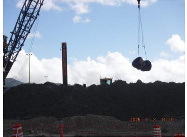
Pier 41: KIWC DB Seattle installing the rubber tire fender skirts around the derrick barge
