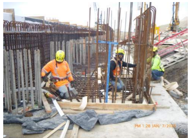
KIWC installing formwork for the power and cable drum vault in WSCRB pour #A5.
