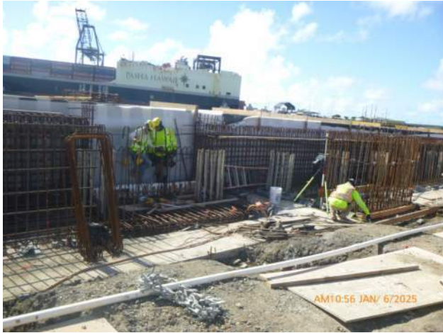
KIWC setting formwork for the cable drum and power vaults in WSCRB pour #A5.
