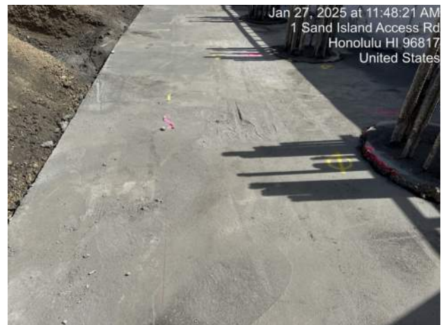
Jan 27, 2025 at 11:48:21 AM 1 Sand Island Access Rd Honolulu HI 96817 United States View of the grinded mud mat of the WSCRb on Pier 43
