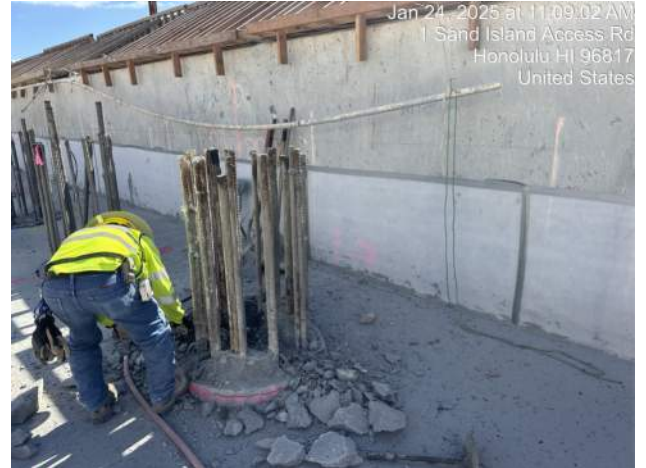
Jan 24, 2025 at 11:09:02 AM 1 Sand Island Access Rd Honolulu HI 96817 United States KIWC performing shaft top prep for CIDH shaft 30-A1-36
