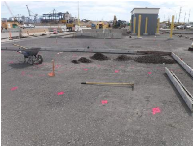
PCCP: MT-10 - KIWC civil crew continued grading the basecourse between 8 and 8.5 inches depth
