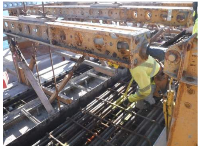
Pier 42: KIWC structure crew adjusted the braces and rebar cage of A3 of the WSCR
