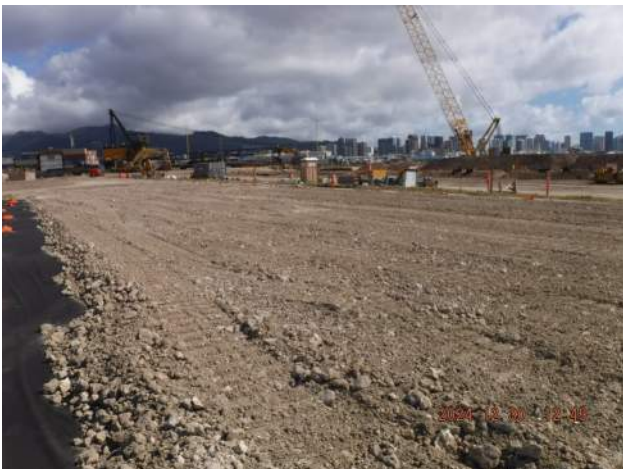
PCCP: KIWC civil crew placed 12-inch thick of the crushed coralline material as a bedding for the future dredged material
