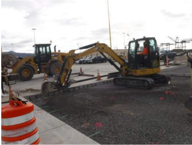
PCCP: KIWC civil crew used the CAT 305 mini excavator to scarify the grade at MT12 (North)
