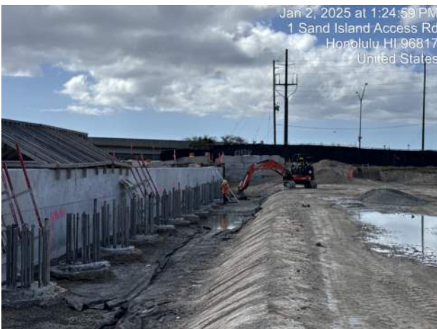
KIWC removing excess concrete and debris from the CIDH installation on Pier 43
