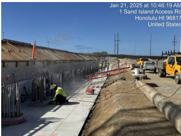
KIWC scoring the edges of CIDH shafts before performing the chipping process for the shafts of the WSCRB
