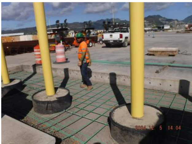
Pier 42: HECO Block Out - HRSPI crew continued installing the rebar mat for the block out
