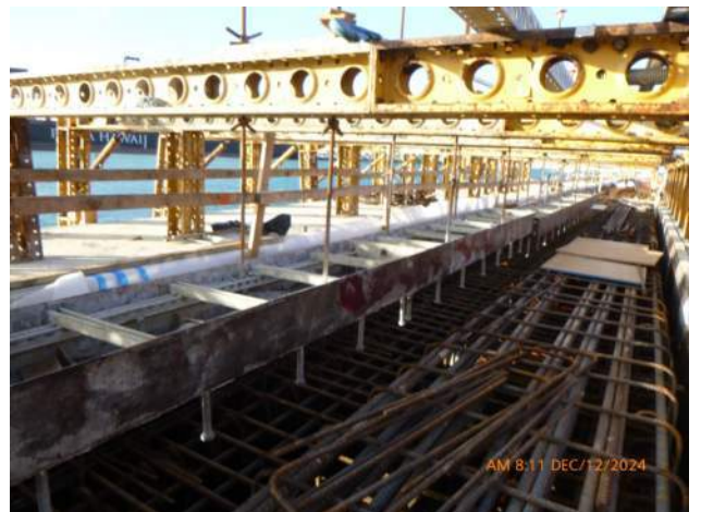
KIWC setting the blackout for the crane rail pocket in WSCRB pour #A3.
