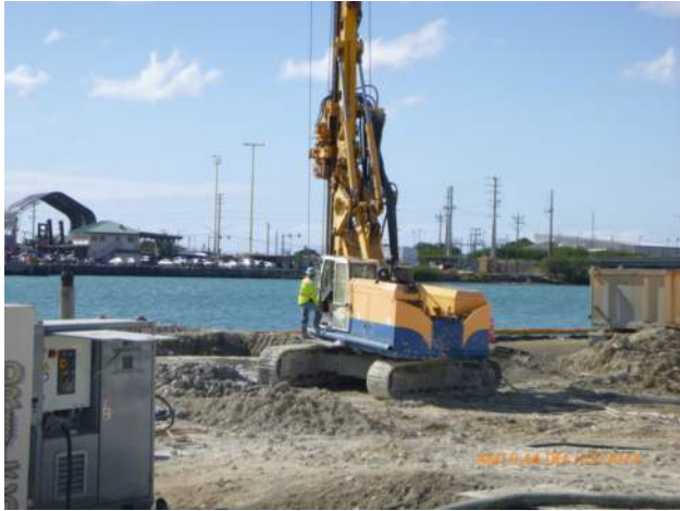
PF jet grouting around the combi wall in the junction structure excavation.
