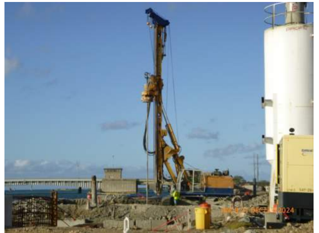
PF jet grouting around the combi wall in the junction structure excavation.
