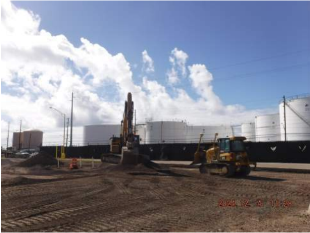
PCCP: KIWC maintenance - KIWC civil crew used the CAT 336 excavator and the CAT D5 dozer to grade the basecourse aggregate
