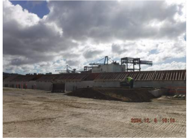
Pier 43: KIWC civil crew continued to construct the platform for coring of CIDH 12-A2-36
