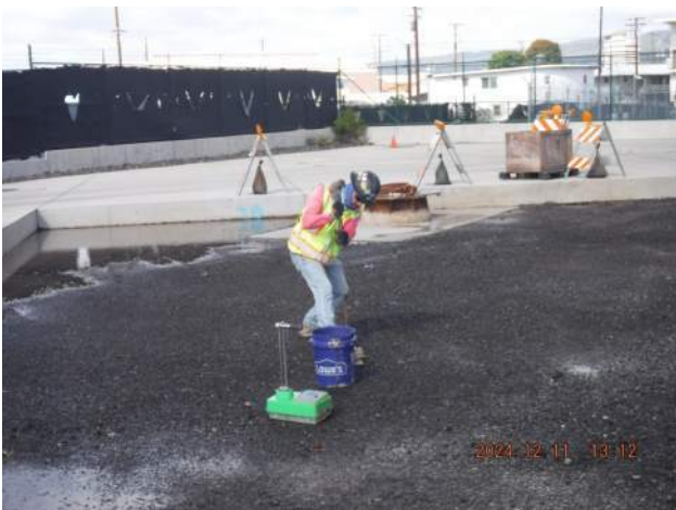
PCCP: PASHA Maintenance block out - MPE tested the moisture content and obtained a dry condition of the subbase
