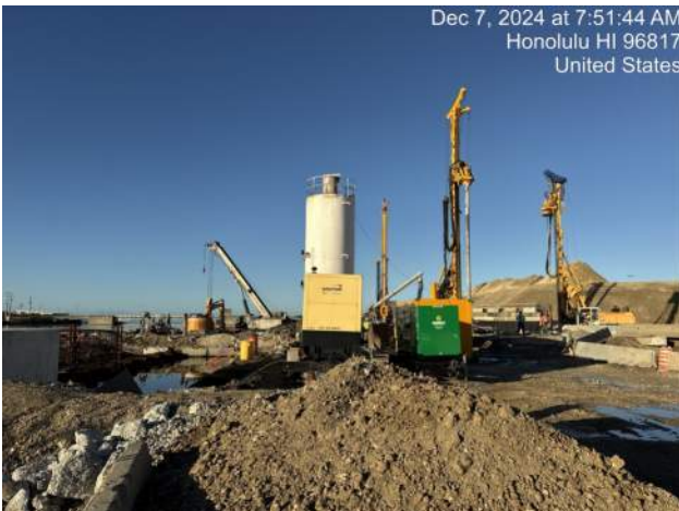
PF on site (using excavator and crane on an object outside of the combi wall)
