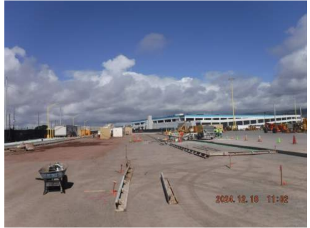
PCCP: Maintenance Shop - Paving crew continued to install the steel forms along the block out
