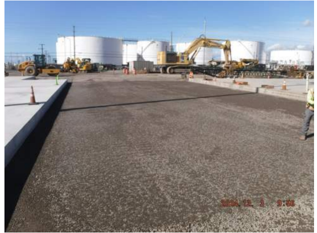
Pier 43: KIWC civil crew continued to fine grade the area on the WL 1 and 2 PCCP blockouts
