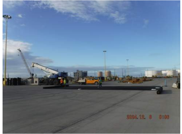
PCCP: KIWC civil crew placing the mirafi fabric for the aeration of the contaminated soil
