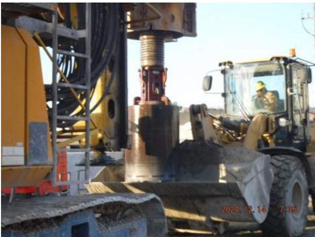
Pier 43: KIWC foundation crew used the clean out bucket to clean the bottom of shaft 12-A1-36
