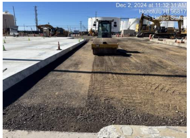
KIWC performing method compaction for the native sub base for the PCCP north of the WMH blockout
