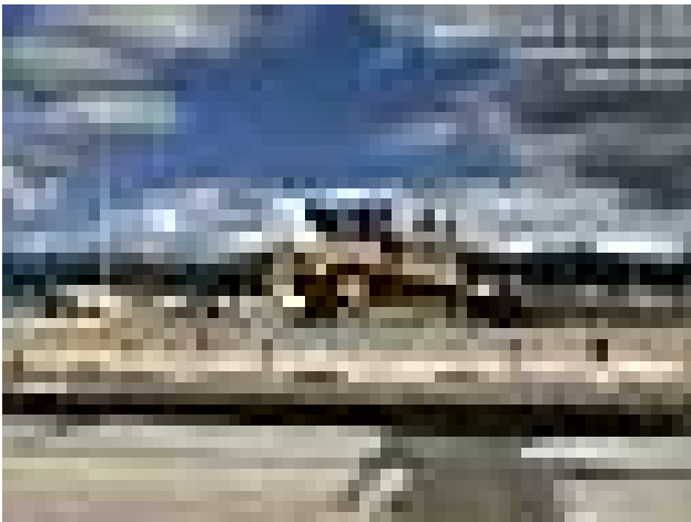
KIWC grading the protective layer on the bottom of the dredge bin on the PCCP at Pier 42
