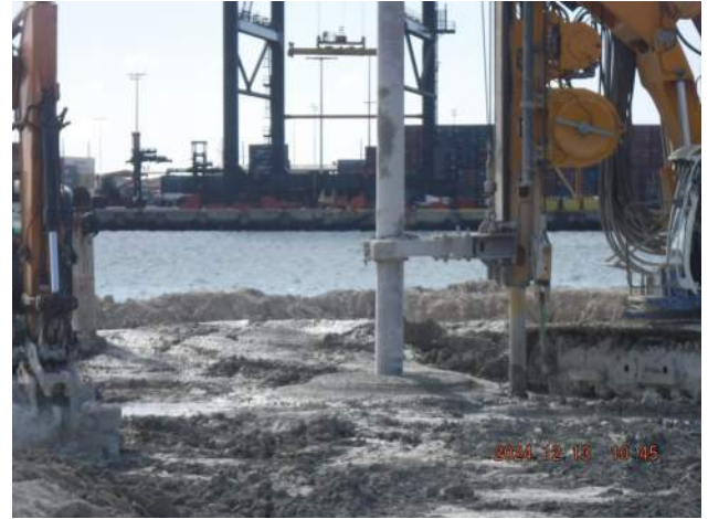
Pier 42: PF continued drilling and soil mixing north of the combi wall of the junction structure
