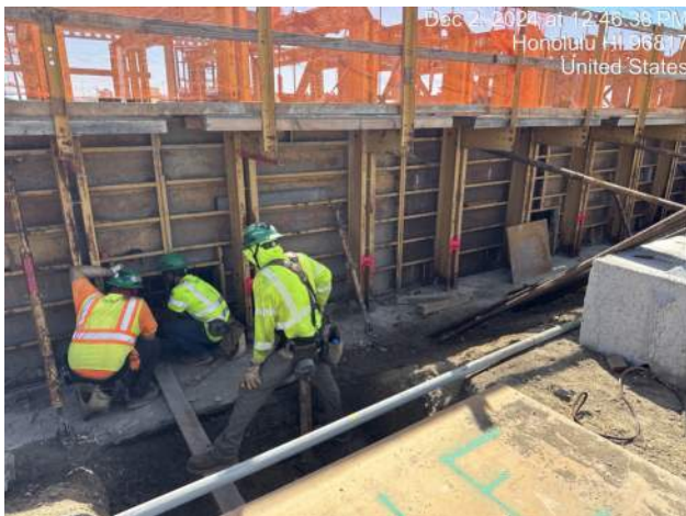
HRSPI installing rebar dowels for the tie beams in pour A2 of the WSCR B
