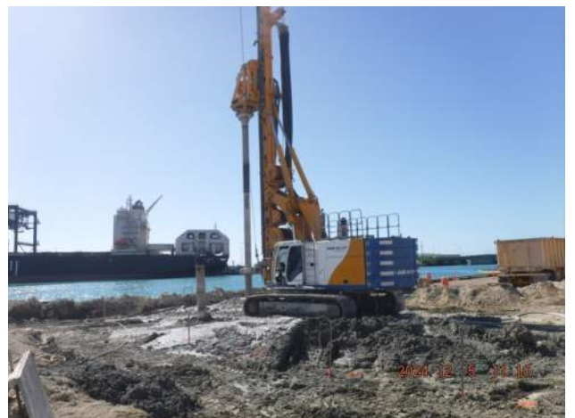
Pier 42: PF crew continued drilling and soil mixing south (outside) the capping beam in the junction structure
