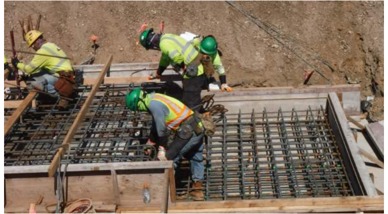
Pier 41: STA 9+00 TD - 3; HRSPI crew continued to install the rebar mat for the floor foundation/invert of the drain inlet
