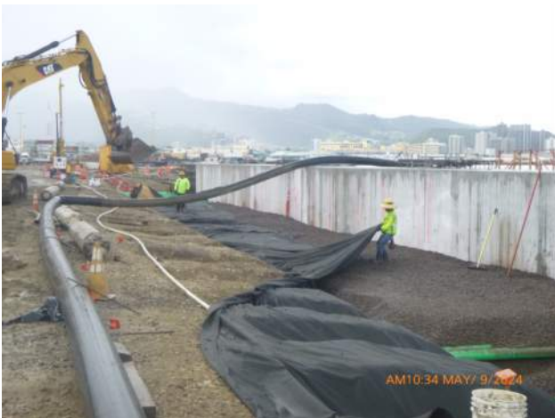
KIWC installing 3b over the tie rods on the landside of the capping beam.
