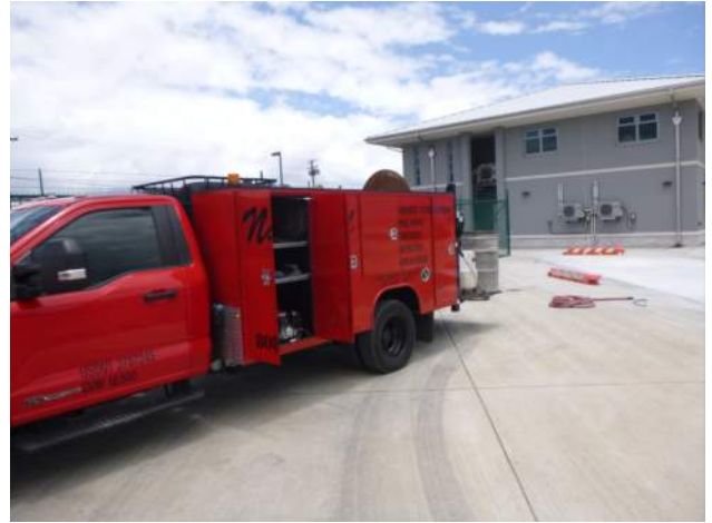
PCCP: National concrete coring on site to green saw cut the newlpy paved area in PASHA maintenance building
