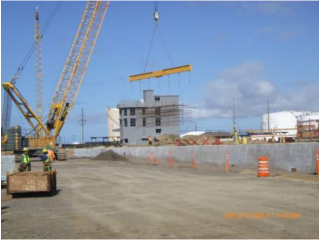
KIWC and HRSPI setting rebar cage for capping beam pour #20 on pier 43.
