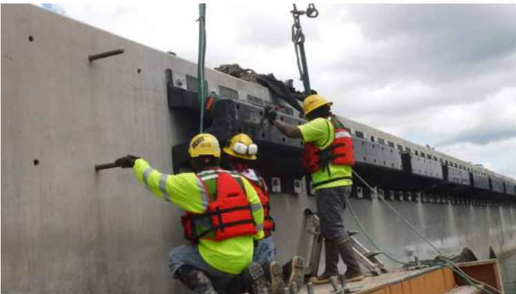
Pier 41: KIWC Bridge and Marine crew used four (4) aligning pins to install the fenders
