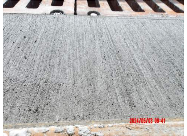
Pier 41: Textured finished of the top of the concrete pour of the trench drain
