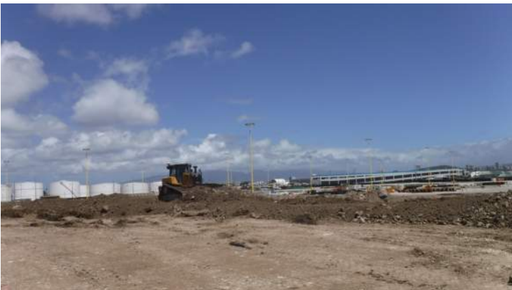
Snug Harbor: KIWC civil crew used the CAT D6 dozer to spread the fill material in 12-inch loose lifts
