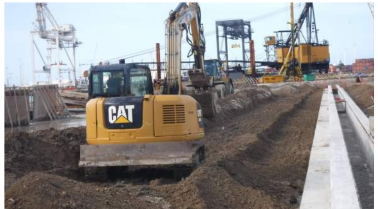
Pier 41: KIWC civil crew continued to scarify and backfill the ocean side of TD-3 wall from STA 1+00 to STA 4+50
