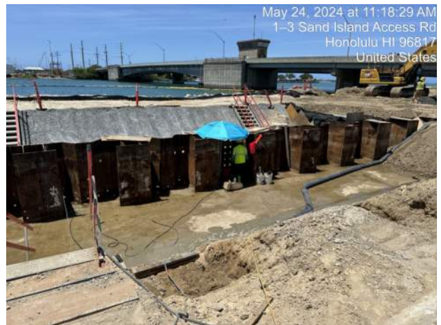
KIWC welding to patch holes burned for the deleted EJ on Pier 43
