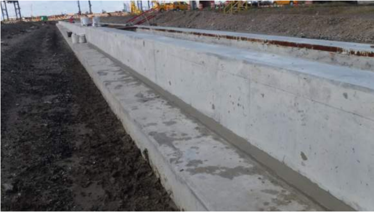
Pier 41: KIWC mason crew continued to patch the honeycombs on the ocean side wall of the trench drain from STA 3+00 to STA 5+00
