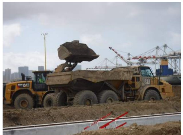
Pier 41: KIWC civil crew continued to haul out the dredged material to Pier 43 stockpile
