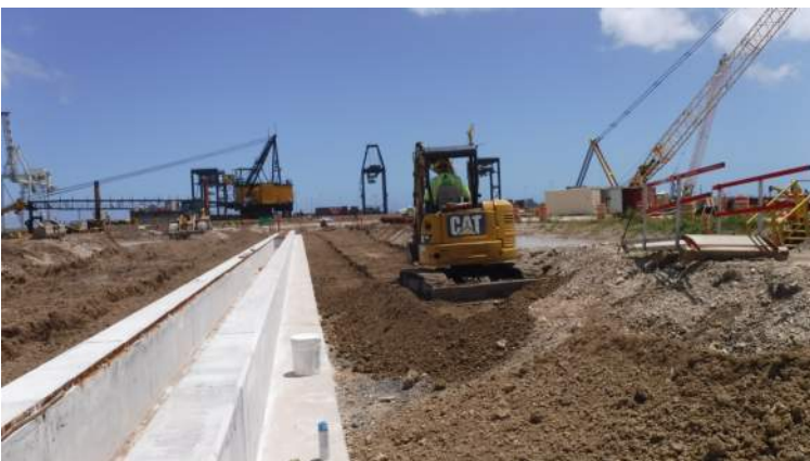
Pier 41: KIWC civil crew continued to scarify and backfill the land side of TD-3 wall from STA 1+00 to STA 4+50
