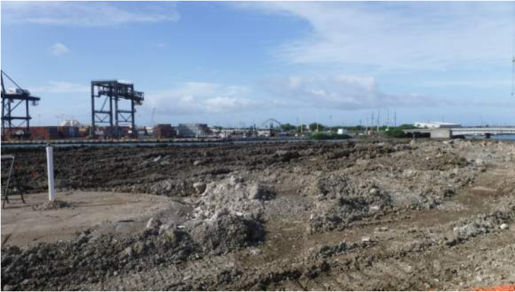
Snug Harbor: ESI personnel on site to collect soil samples for the 19th lift of the surcharge
