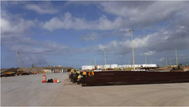
PCCP: HRSPI crew continued to correct the rebar laps for the 36-inch rbar cage
