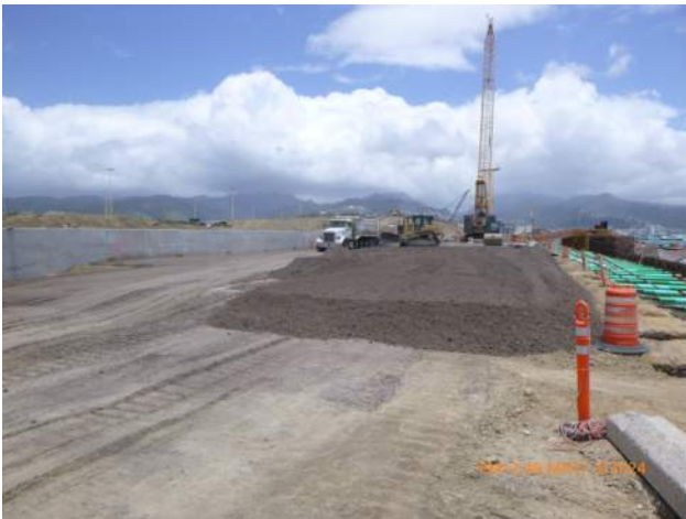
KIWC grading the area between the LSCRB and the combi wall on pier 43.
