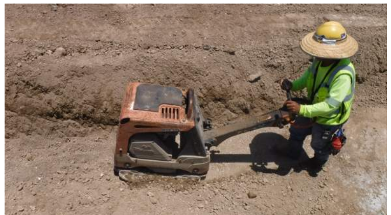
Pier 41: KIWC civil crew used the Mikasa MVH 408 vibratory steel plate to compact the fill on the east side of the trench drain
