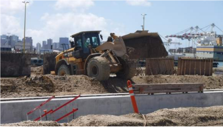
Pier 41: KIWC civil crew continued to backfill the ocean and land sides wall of the trench drain from STA 1+00 to STA 4+00
