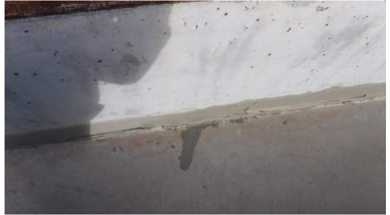
Pier 41: KIWC mason crew continued to patch the honeycombs in the inner walls of the trench drain
