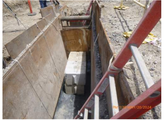
KIWC setting formwork for the CLSM pour on the ends of the W-2 excavation.
