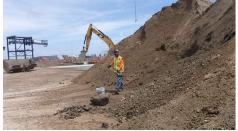
Pier 43: Collected soil samples for Proctor and gradation tests from P7/P8 LSCRB mass excavation
