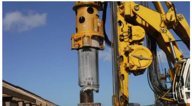
Pier 42: KIWC Foundation crew used the drilling bucket to drill the shafts
