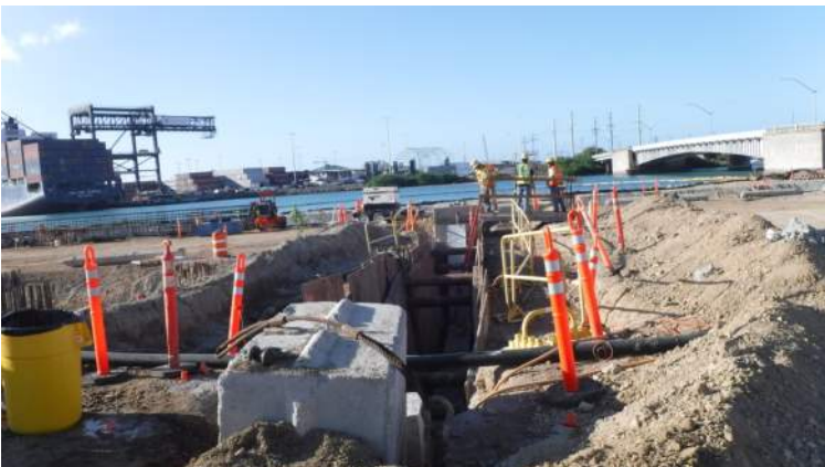
Pier 43: KIWC civil crew (Micah's) cleaned the bottom of WL-2 before placing #3B fine gravel
