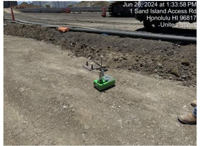
MPE performed compaction test of lift 2 of P18 of the cap beam backfill (results in question due to results not matching the proctor)
