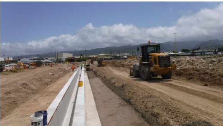
Pier 41: The Sakai SW300 double drum vibratory roller was used to compact the backfill material on the east side of the trench drain
