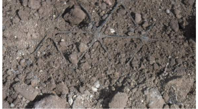
PCCP: PASHA maintenance building - KIWC civil crew (John's) pot holed and exposed the location of the geogrid
