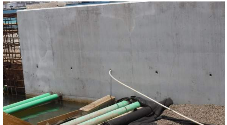
Pier 42: KIWC mason crew grouted the form tie holes of P14 of the CWCB
