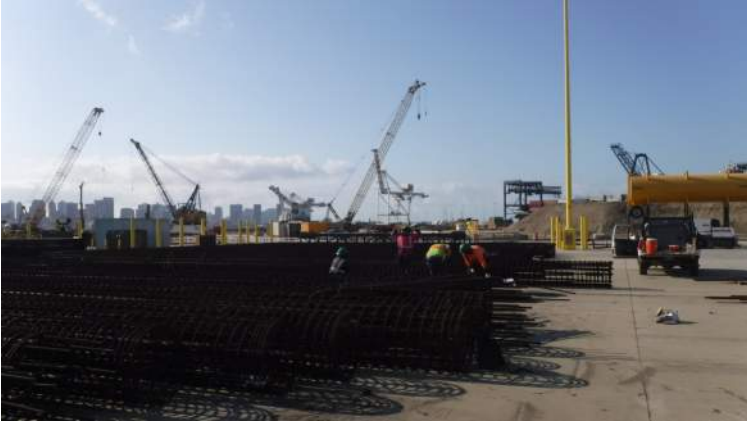
PCCP: HRSPI crew continued to correct the rebar laps for the 36-inch CIDH cage
