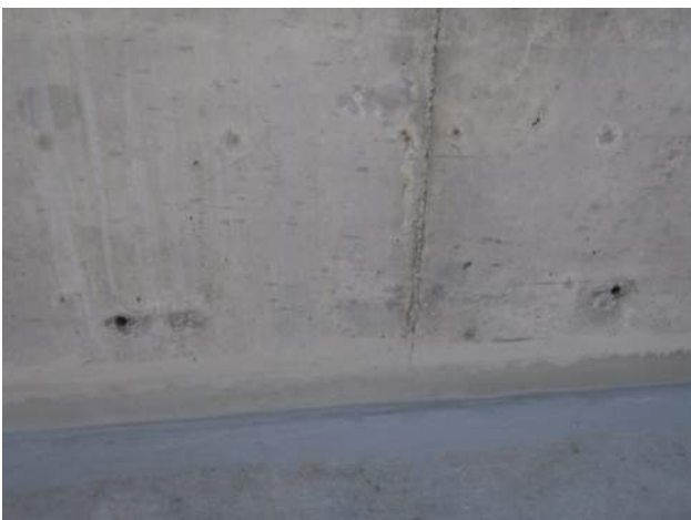
Pier 41: KIWC mason crew continued to grout the form tie holes of trench drain 3
