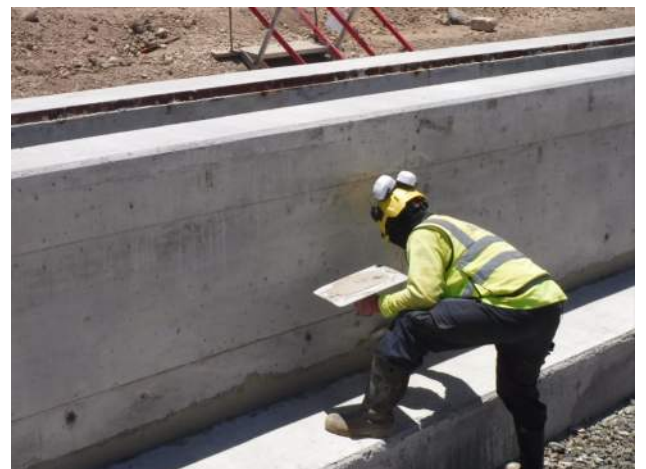
Pier 41: KIWC mason crew continued to grout the form tie holes of trench drain 3
