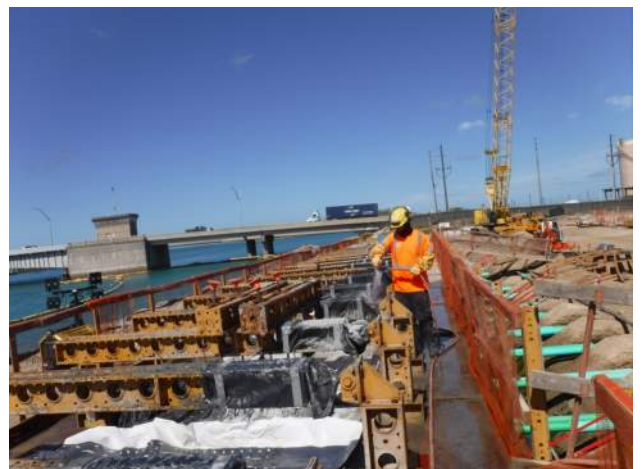
Pier 43: KIWC mason crew applied concrete curing compound for pour #P21 of the CWCB
