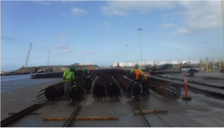
PCCP: HRSPI crew continued to correct the rebar cage of the 36-inch CIDH
