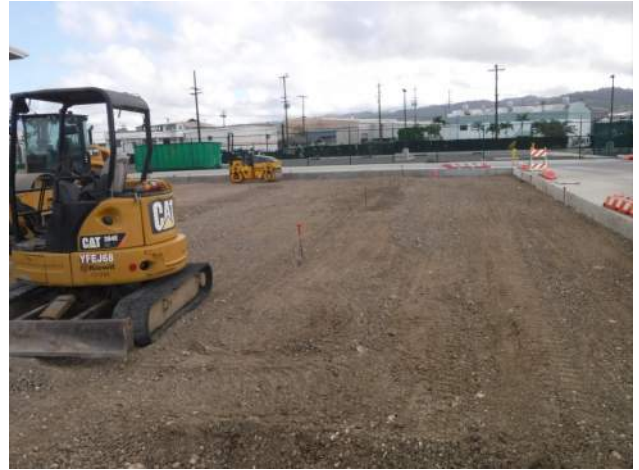
PCCP: PASHA- maintenance building; The crew used the CAT 305 mini excavator to fine grade the block out
