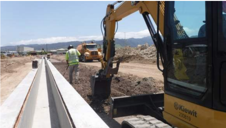
Pier 41: KIWC civil crew continued to use the CAT 305 mini excavator to scarify the fill from STA 4+00 to STA 4+50
