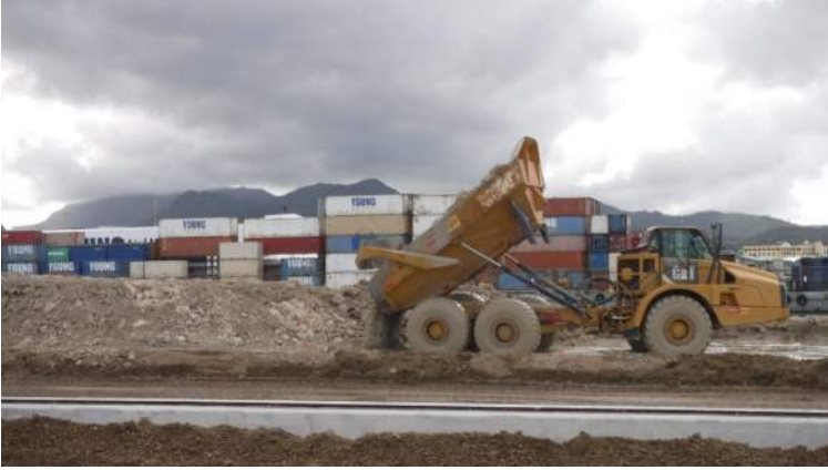
Pier 41: KIWC Bridge and Marine crew used the CAT 740 rock truck to unload the dredged material into the stockpile
