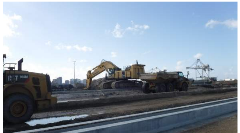
Pier 41: KIWC Bridge and Marine crew unloading the dredged material from the dump scow
