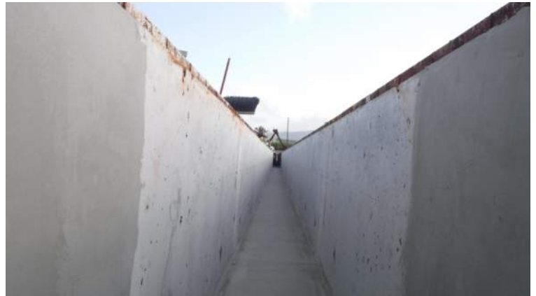
Pier 41: KIWC mason crew continued to concrete dry finished the inner walls of Trench Drain 3
