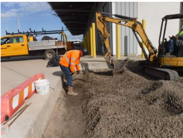
PCCP: PASHA maintenance building - The civil crew (John's) crew continued to scarify the existing subgrade to remove the damaged geogrid
