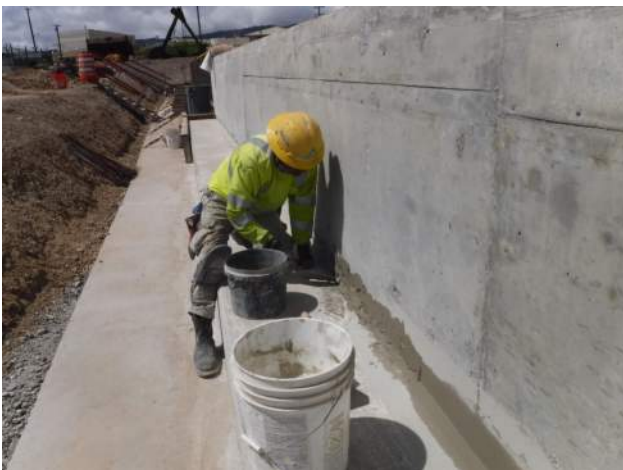
Pier 41: KIWC mason crew continued to patch the honeycombs of the exterior wall of P7 of the trench drain
