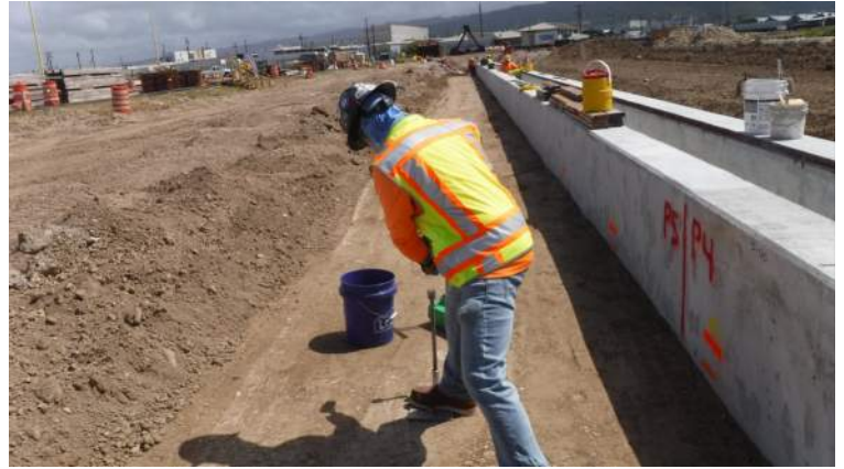
Pier 41: MPE soil technician took density tests of the compacted fill for the third lift
