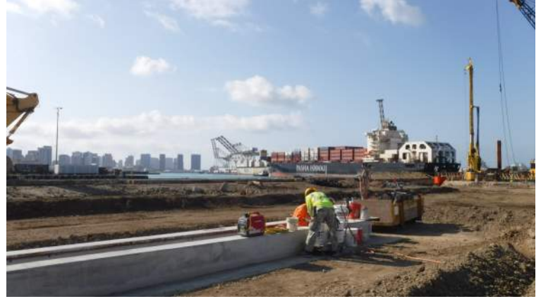
Pier 41: KIWC mason crew continued to patch the inner walls of the trench drain from STA 1+00 to STA 2+00
