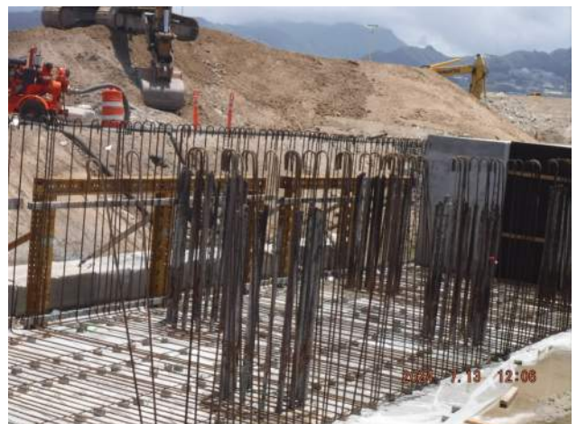
Pier 43: HRSPI crew continued installing the "U" rebar mat and wall cage for P7/P8 of the LSCRB
