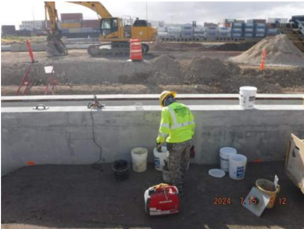
Pier 41: KIWC mason crew continued to patch the honeycombs inside the inner wall of the P7 of the TD - 3
