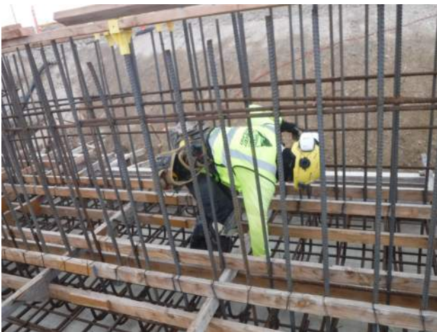
Pier 41: KIWC carpentry crew continued to conduct rebar corrections of P8 of the trench drain
