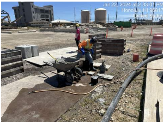
MPE testing truck 1 of the CIDH shaft pour (no shafts ended up being poured this shift)
