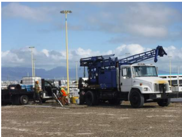
Snug Harbor: KGI on site to mobilize to boring 102 of the surcharge fill
