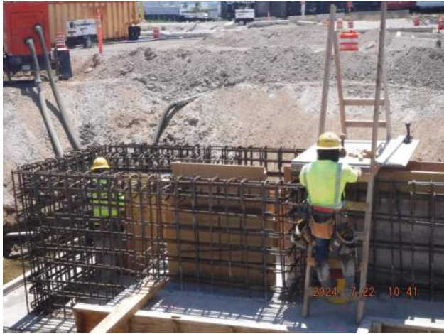
Pier 41: KIWC carpentry crew continued to install the forms for the drain inlet and P8 of the trench drain
