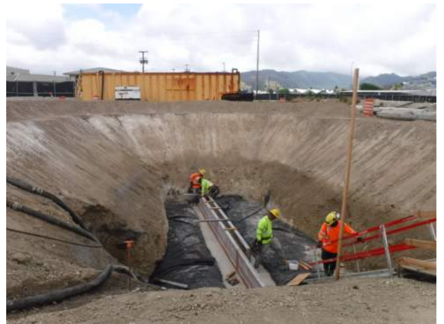
Pier 40F: KIWC carpentry crew fabricated the keyway for the storm drain headwall
