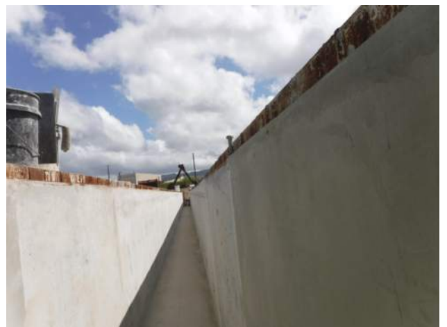
Pier 41: KIWC mason crew continued to concrete dry finish the interior wall of P7 of the trench drain
