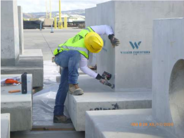
KIWC wire wheeling the surface of the SDMH's staged on the PCCP.
