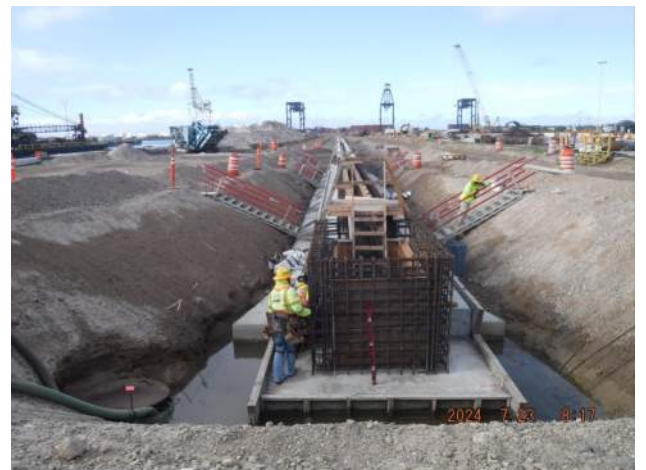
Pier 41: KIWC carpentry crew prepared P8 of the trench drain 3 and the drain inlet for structural observations
