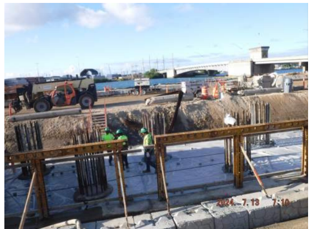
Pier 43: HRSPI crew on site installing the rebar cage for P7/P8 of the LSCRB
