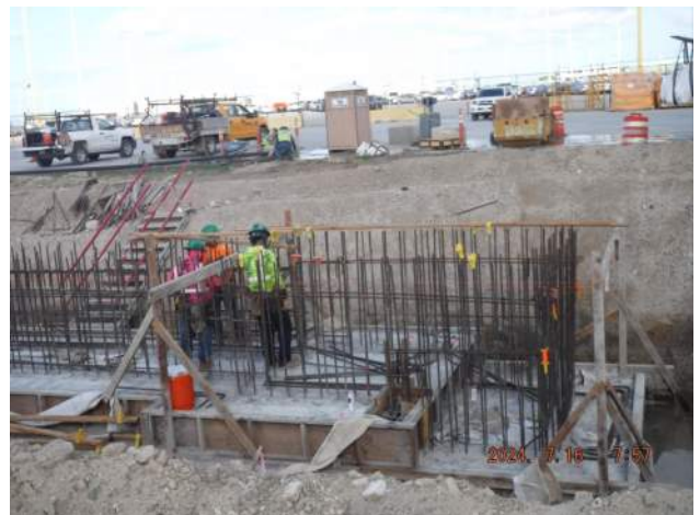
Pier 41: HRSPI crew continued installing rebars for the walls of P8 and drain inlet of the TD 3
