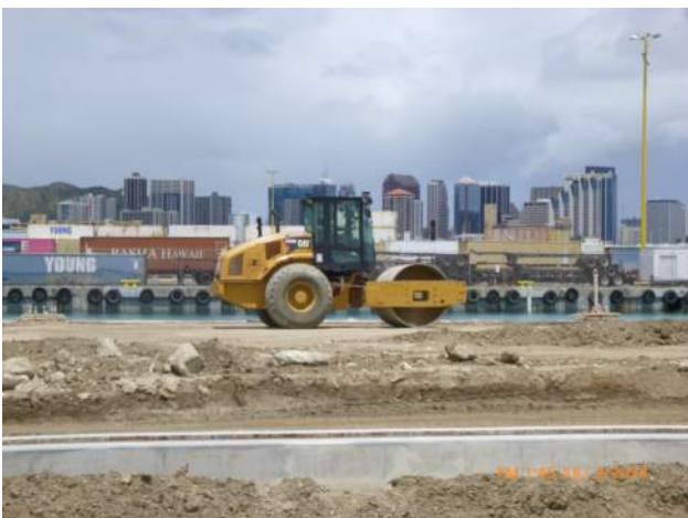
KIWC building up the grade on the landside of the capping beam.
