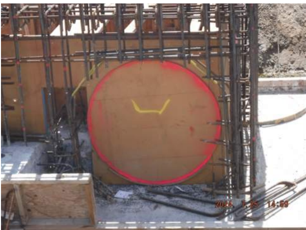
Pier 41: HRSPI crew cut the rebars for the 36-inch RCP block out of the drain inlet of Trench Drain 3
