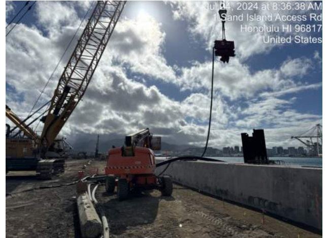
KIWC prepping to remove the temporary sheet piles on the waterside of the cap beam
