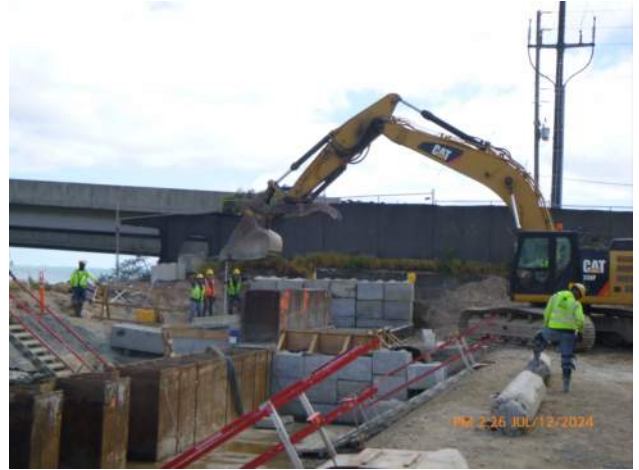
KIWC pouring the mud mat around the end of the continuous king pile wall.
