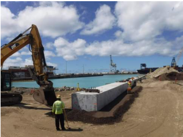
Pier 41: KIWC civil crew (Sanu's) continued to use the Mikasa MVH 508 vibratory steel plate to compact the fill placement
