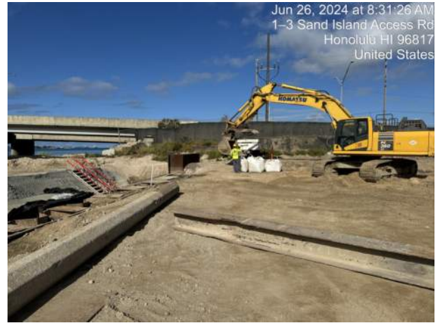
KIWC prepping to excavate and grade the area for installation of P25 of the cap beam on Pier 43
