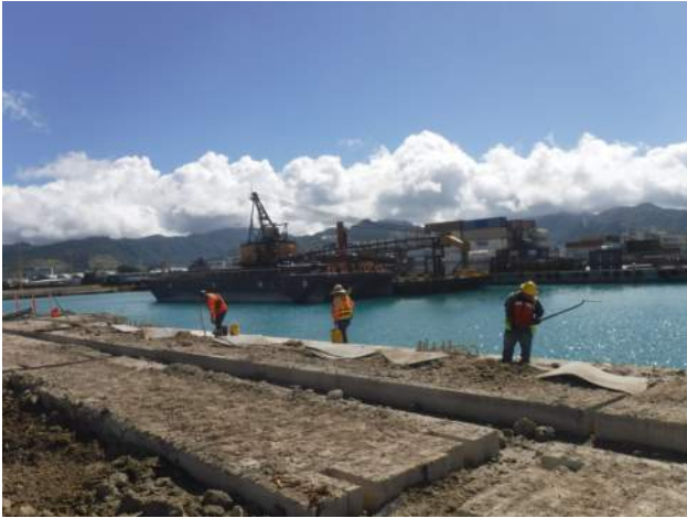
Pier 41: KIWC civil crew removed and cleaned the top of the capping beam from STA 19+00 to STA 21+00 of the dredged spoils
