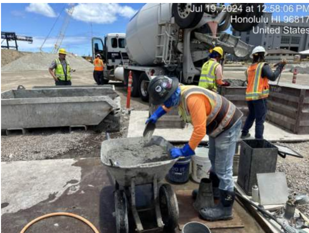
MPE testing the concrete for truck 3 of the CIDH shaft installation due to trucks 1 and 2 timing out
