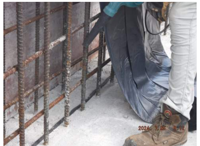
Pier 41: KIWC carpentry crew used hand blower to remove concrete stones between the vertical rebars
