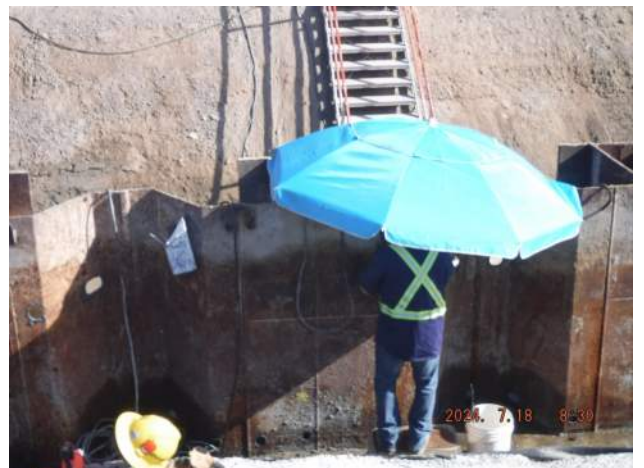
Pier 43: KIWC welder welded the "U" rebar between the king and sheet pile interlocks of P24 of the CWCB
