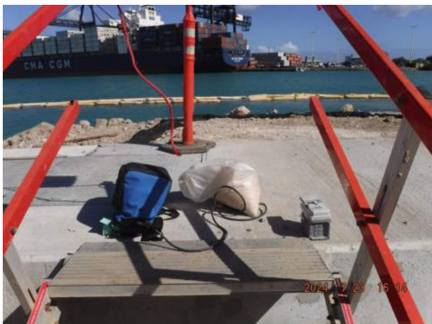
Pier 43: Vibration monitoring instruments placed over the CWCB of P16
