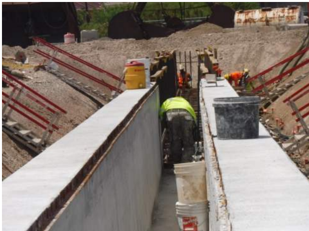
Pier 41: KIWC mason crew continued to patch the honeycombs inside the inner wall of the P7 of the trench drain
