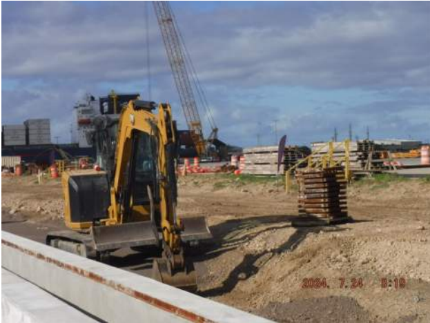
Pier 41: KIWC carpentry crew continued to install the grates for the trench drain 3
