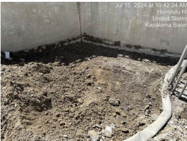
View of KIWC progress performing shaft top prep of the WSCRB on Pier 42
