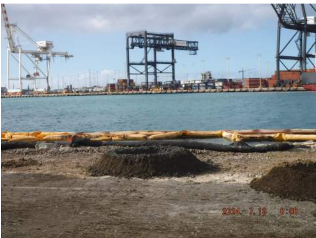
Pier 42: The foundation crew drilled and probed for obstruction at the junction structure drain outfall
