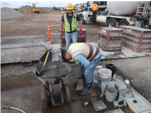
Pier 41: MPE tested the concrete parameters of the first load of concrete truck mixed - Temp: 86 deg F, slump: 5.25", air content: 3.3%
