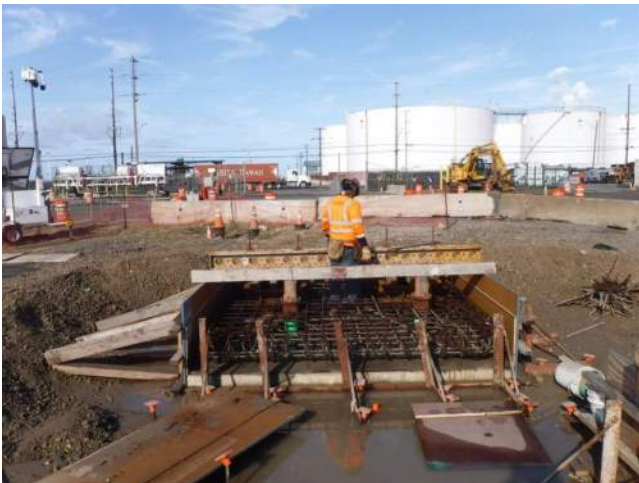
Pier 43: WL 1 and 2 - HRSPI crew continued to rework the steel cages for the water manhole covers
