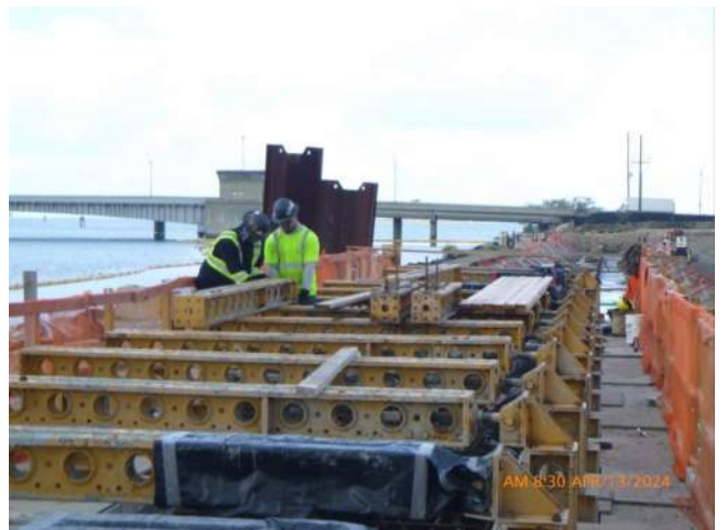
KIWC adjusting supports for the shore power vault in capping beam pour #16.
