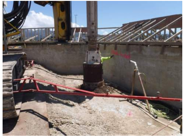
Pier 42: Location of CIDH drilling for # 59-A4-36 shaft on P1 of the CWCB
