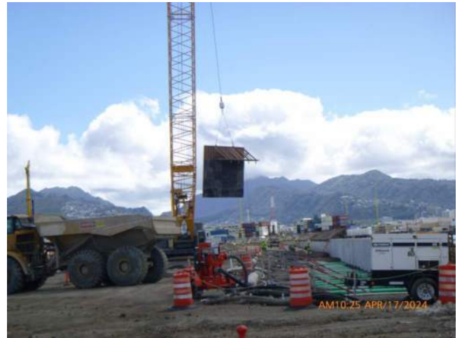
KIWC placing dredging panels over the waterside of the pier 42 capping beam.
