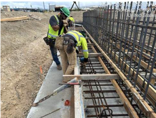
HRSPI installing 3" dobies to achieve 3" cover for the reinforcement of TD-3 P7B
