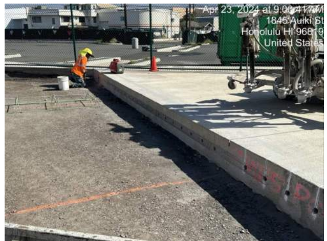
KIWC finishing drilling for installation of dowels for the north breakout at the PASHA maintenance building
