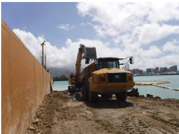
Pier 42: KIW civil crew continued in land water dredging on the ocean side of P4 and P5 of the CWCB
