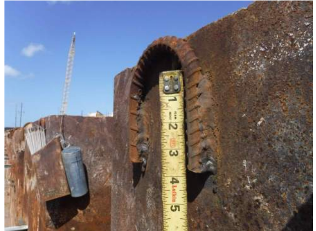
Pier 43: KIWC welder welded the #8 "U" rebar between the sheet and double king pile interlocks from P20 to P21 of the CWCB
