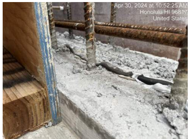
KIWC finished chipping the excess concrete on the waterside of TD-3 Sta. 7+94 to 8+00
