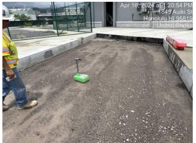
KIWC scarified and compacted the utility trench area of the north maintenance building blackout
