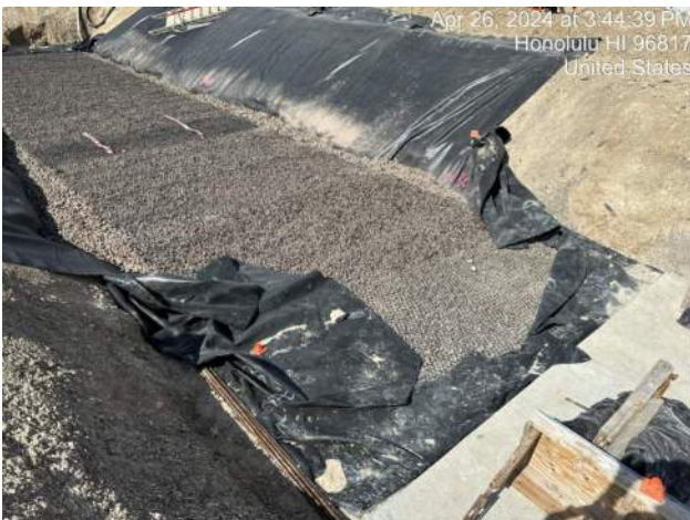
KIWC placed third layer of geogrid for TD-3 stabilization layer from Sta 8+00 to 9+00
