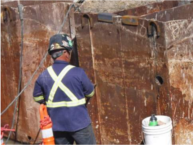
Pier 43: KIWC welder continued to weld the waler braces between P20 and P21 of the CWCB
