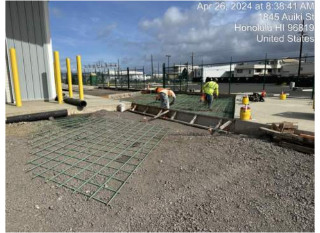
KH observed KIWC installing the formwork and rebar mats for the PASHA maintenance building north breakout
