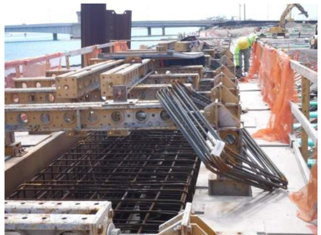
Pier 43: HRSPI crew was on site for install the rebar cage for the shore power vault in P16 of the CWCB
