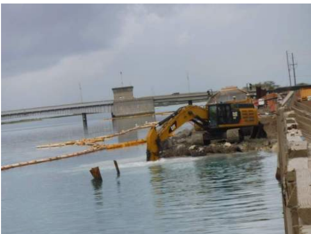
Pier 42: KIWC civil crew continued to conduct in-land water dredging on P6 of the CWCB
