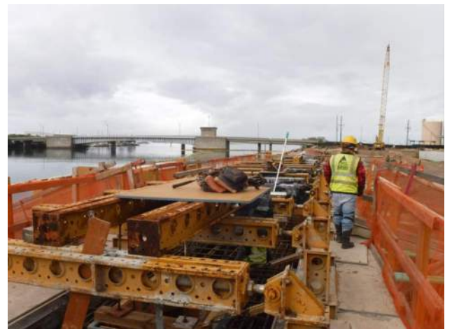
Pier 43: KIWC carpentry crew continued to set the forms for the EJ of P17/P18 of the CWCB
