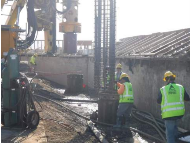
Pier 42: KIWC foundation crew set up the CIDH cage into CIDH #56-A4-36
