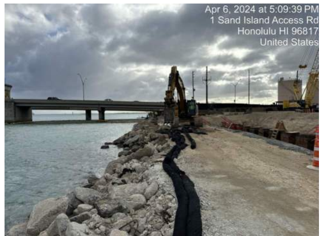
KIWC fully removed the material placed for stone column installation on Pier 43
