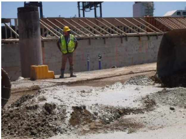
Pier 42: The grades changed to tan to white coralline sandy silt and gravel at 30 to 45' bgs
