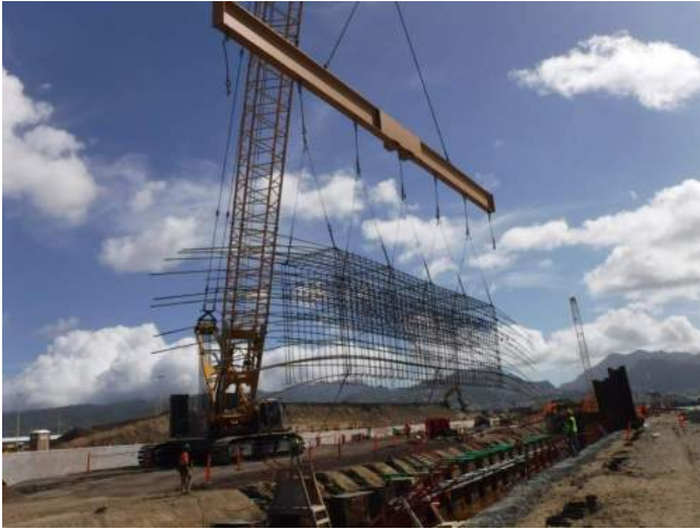
Pier 43: HRSPI crew on site to install the rebar cage for P17 of the CWCB
