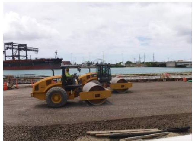
Pier 43: Two CAT CS 56 vibratory rollers were used to roll the fill placement by Method Compaction on P4 of the LSCR B
