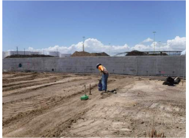
Pier 43: MPE soil technician to test the density of the compacted fill between P4 and P5 of the LSCRB
