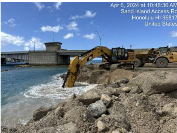
KIWC performing landside dredging to remove KIWC's previously placed fill on the waterfront of P43
