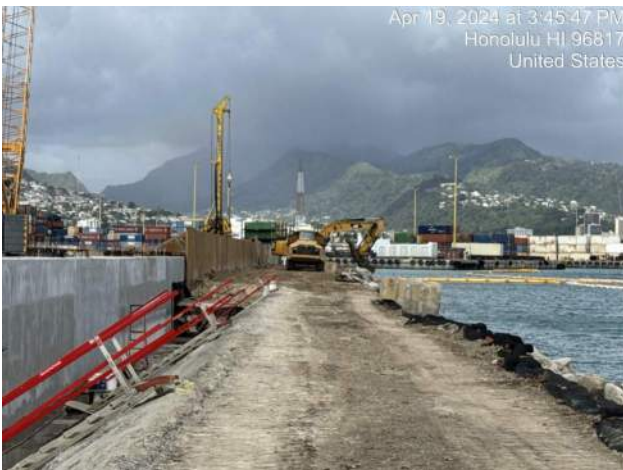
KIWC started the landside dredging on Pier 42 using the CAT 349F excavator
